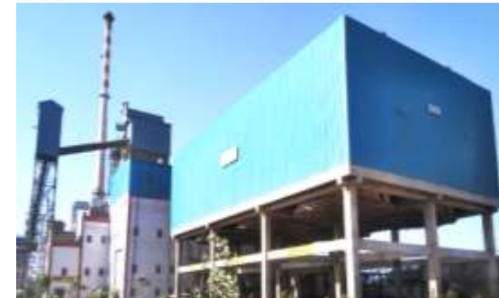
AIR COOLED CONDENSER
