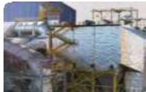
Air Pollution Control
